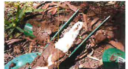
Photo 1: Partially consumed termiticide rod which needs replacing.
